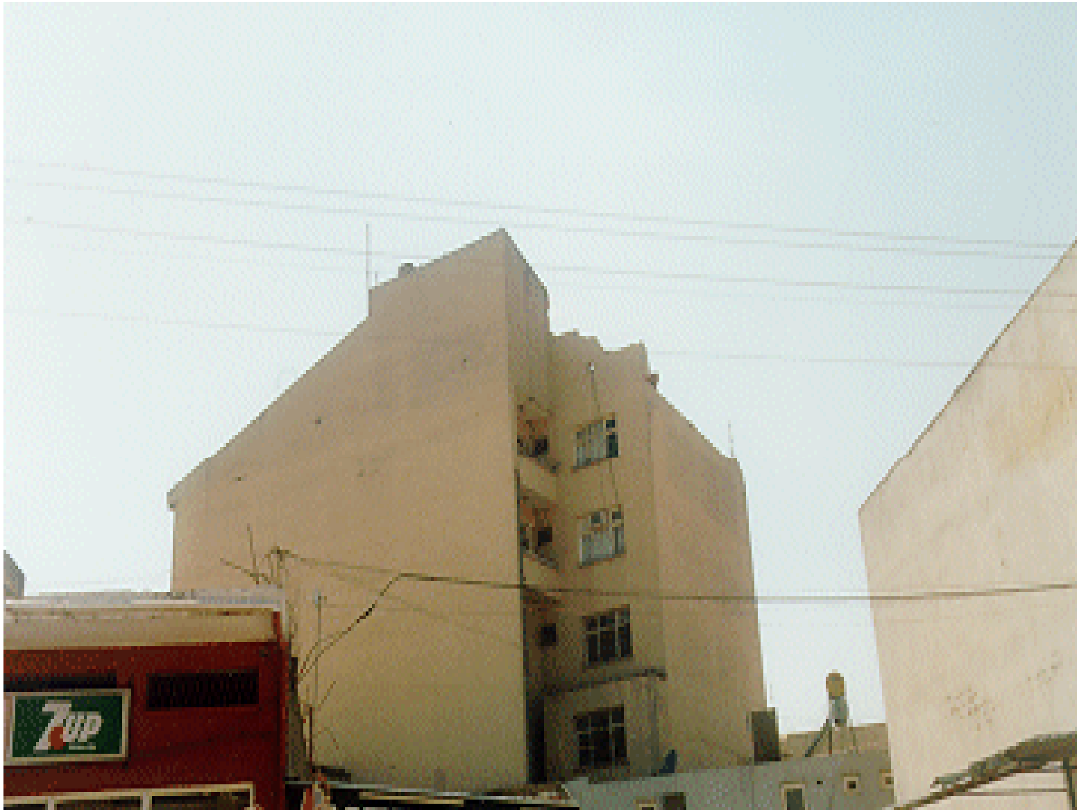
Collapsed Gable and Parapet Wall of The Police Headquarters ( Bayulke,1998 )
